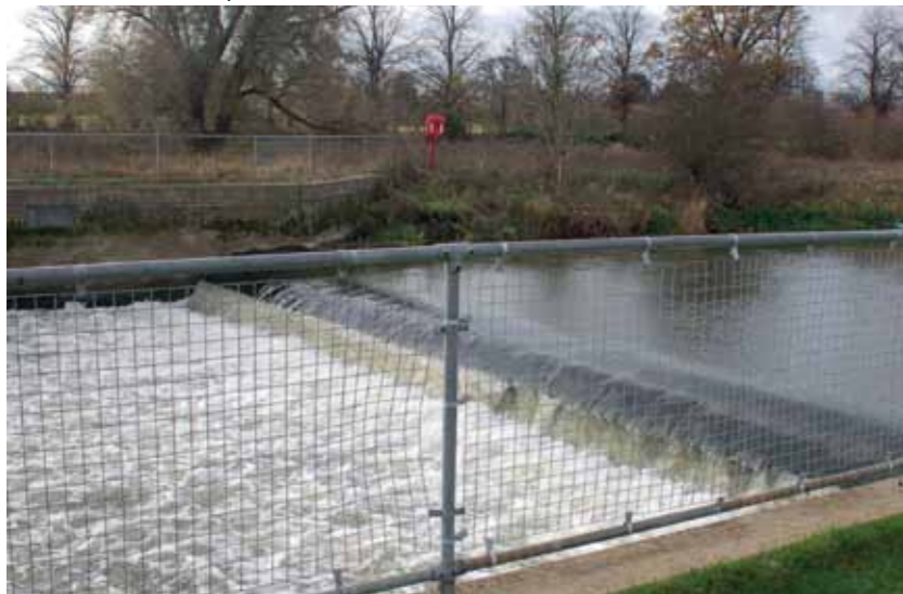
MEDIUM FLOW Note sturdy fence to restrict public access and rescue ring on the far bank to lower risks
