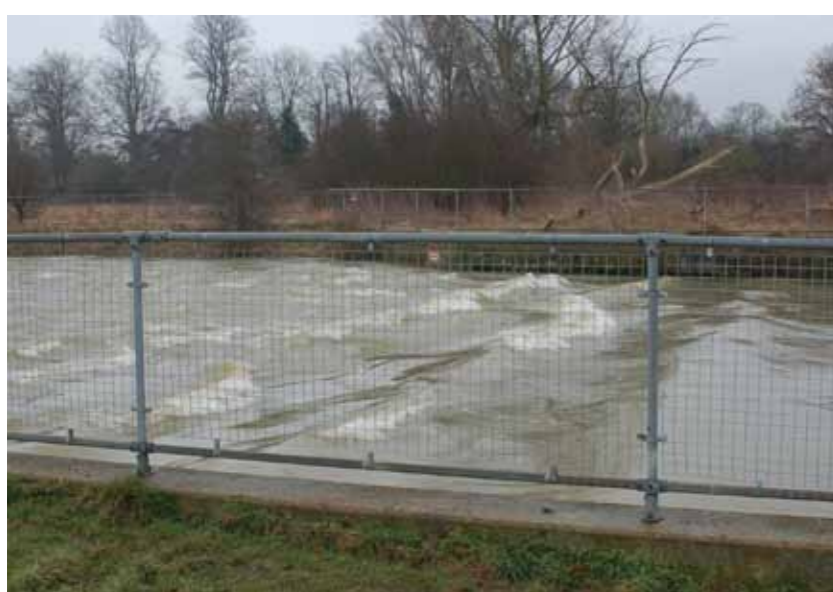
HIGH FLOW. Weir is washed out by high water volume
